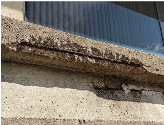
Spalled concrete slab edge/exposed rebar
