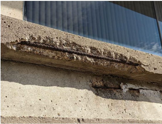
Spalled concrete slab edge/exposed rebar
