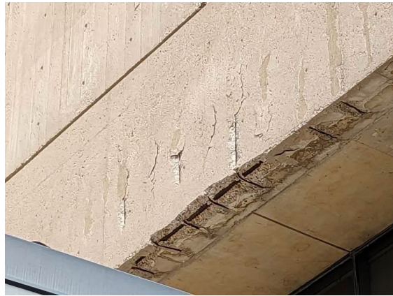
Concrete vertical surface spalling
