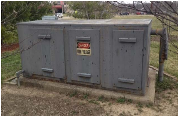
Current 'Pad Mount' Loop Switch
